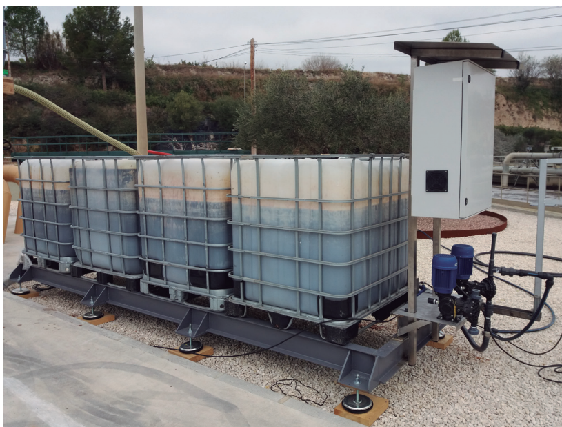
FIGURE 2. Dosing system installed at Ontiyent-Agullent WWTP
